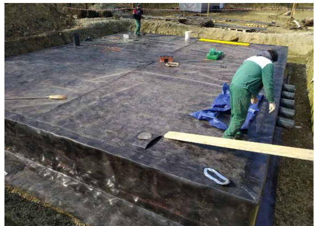
A retention with dimensions 10.8 x 9.0 x 0.9 m and volume of 85 m 3 , is installed under the customers car parking area. The thickness of the cover (backfill soil and the upper road structure of the parking area) is 1.4 m.
